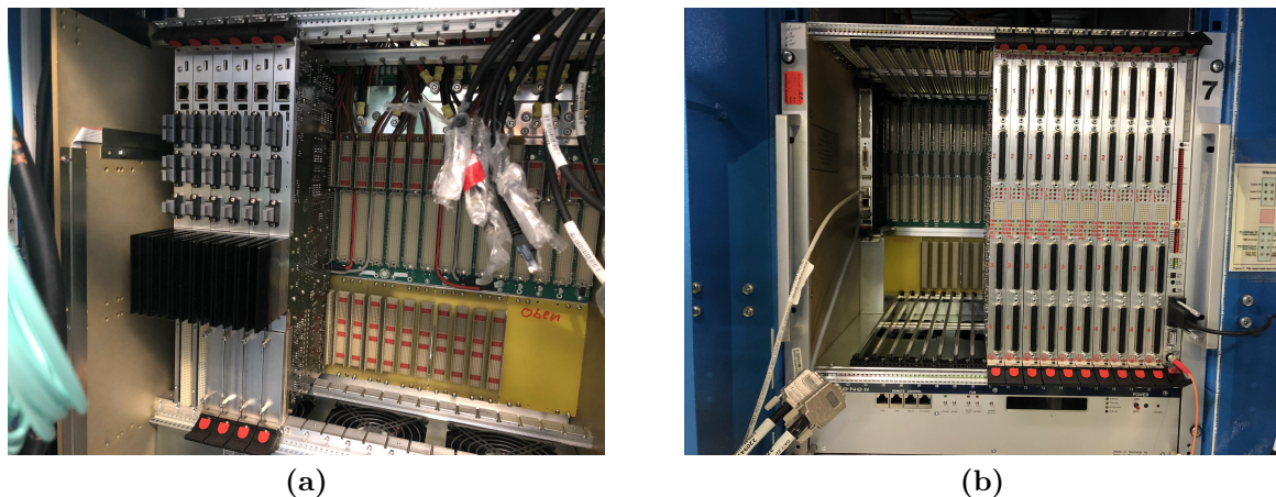
Figure 8.1. The back view (a) of the VME crate with TREX modules inserted. The frontal view (b) with PPMs re-inserted after the hardware adaptations.
